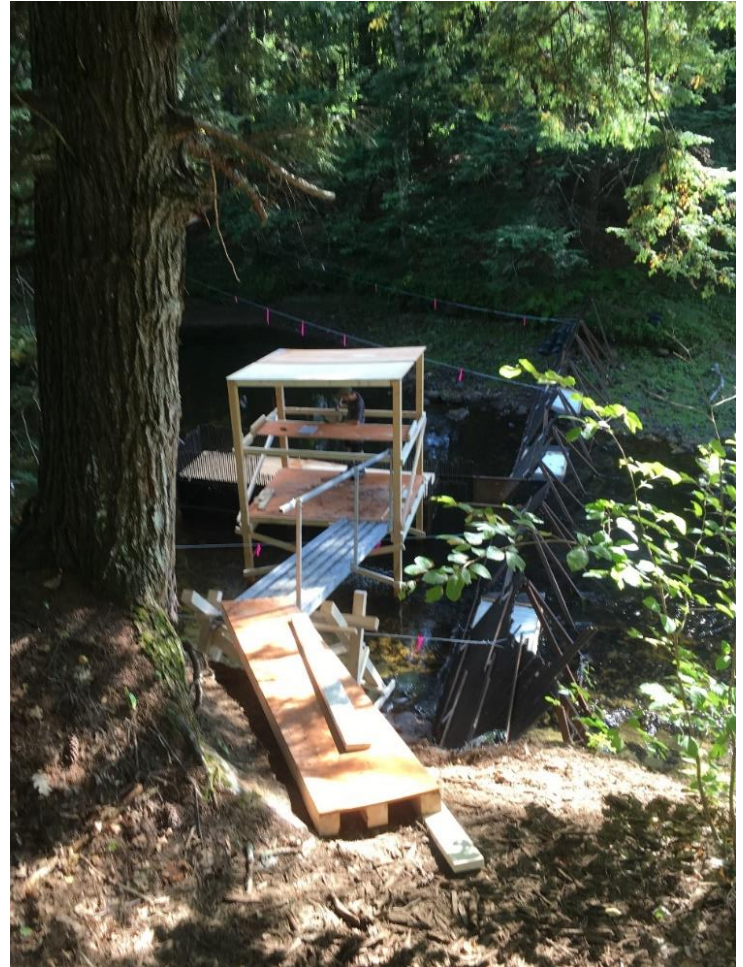
Figure 3. Work platform and access walkway descending from the riverbank to the weir collection box.
